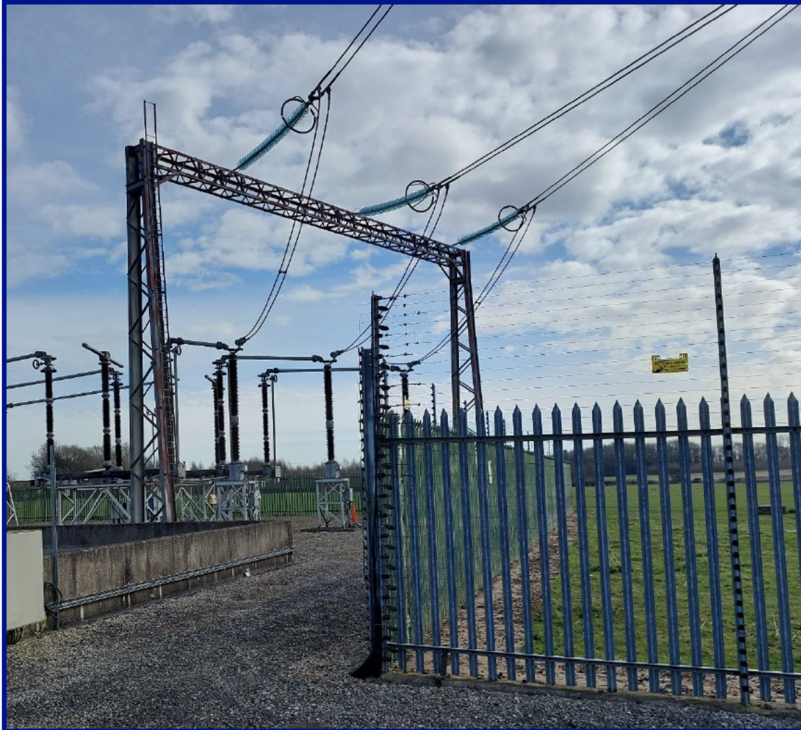
Figure 4: Existing CSE with gantries (Source: MM Site Visit)
